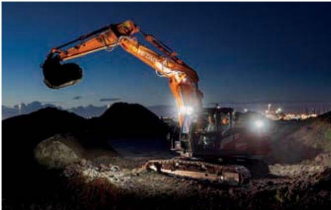
LED work lights improve visibility in challenging conditions.
